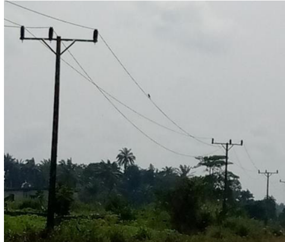
Figure 4: Sagging transmission cables Between Oleh and Ozoro community.
