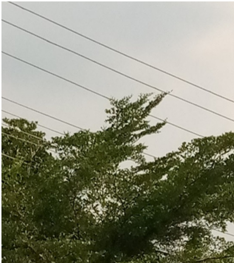
Figure 5: Secondary distribution line overgrown with trees.
