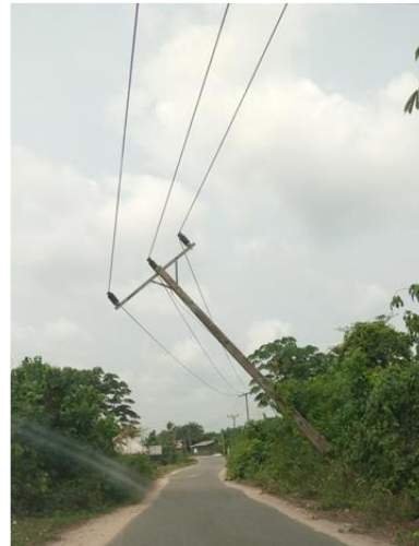
Figure 6: A slanting utility pole at Owhe community
