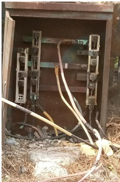
Figure 7: A transformer feeder pillar.
