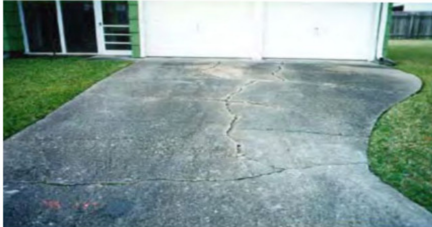
Figure 10: Residential driveway damaged by expansive soil (Al-Homoud et al. , 1995).
