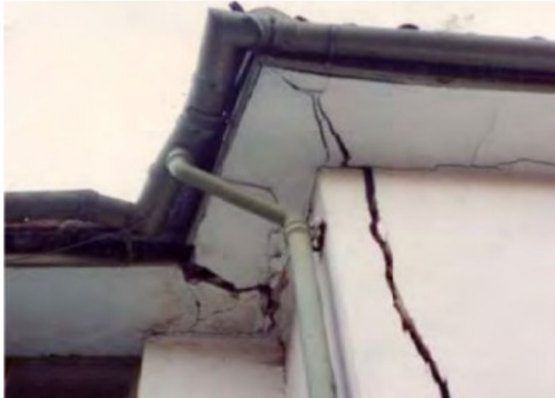
Figure 8: Structural damage to house caused by 'end lift' (Lee, 2011).
