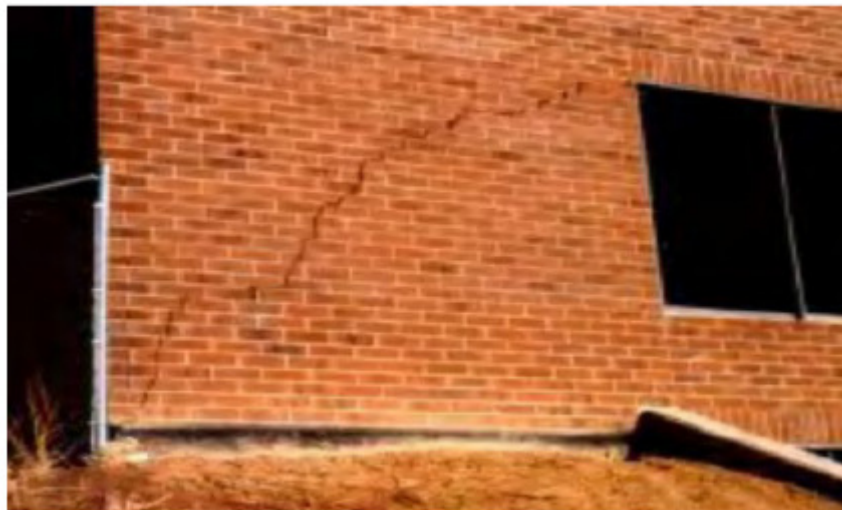
Figure 9: Major cracks in exterior walls at doors and windows (Gunev et al, 2007).
