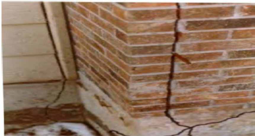
Figure 11: Cracks in exterior walls, as a result of upward soil expansion (Popescu, 1980).
